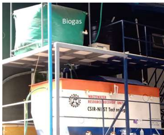
NOWA unit installed in a medium scale industry recovering reuse quality water and biogas from wastewater.
