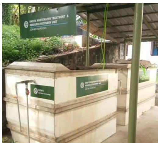
NOWA unit installed in NIIST campus treating 10 KLD wastewater from NIIST canteen.
